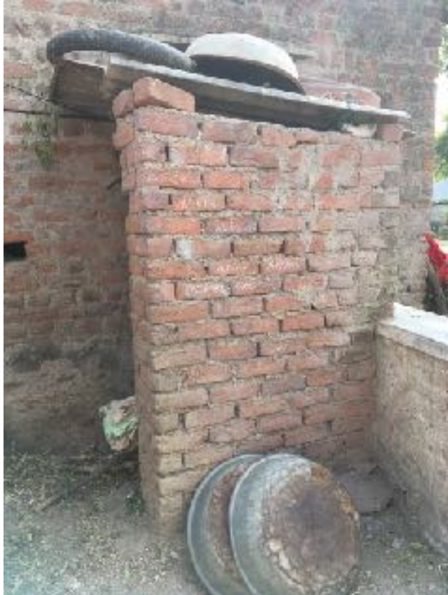
Figure 7: A government-constructed latrine in Umarni Village with a makeshift roof.
