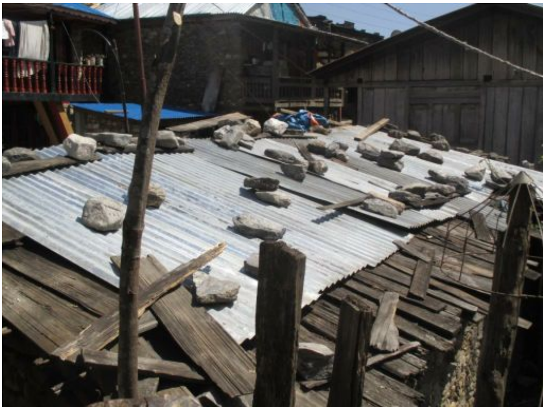
Picture 17: Tin roof held in place by rocks
