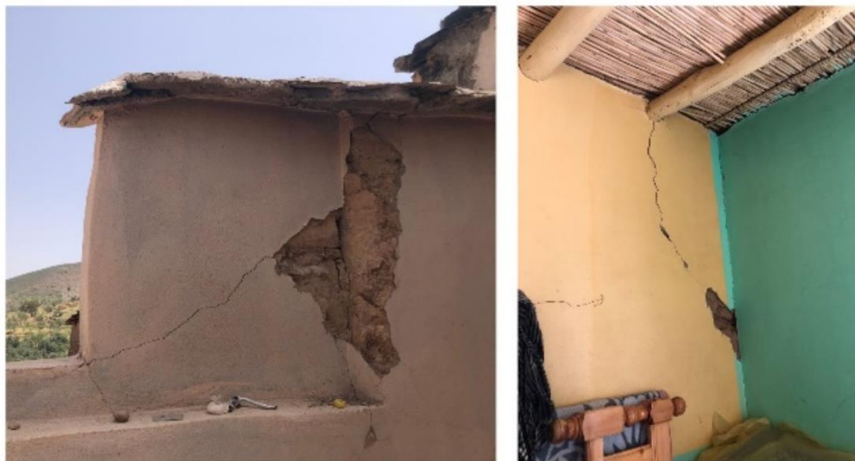
Figure 1.2. Ait Bourde damage to resisting infrastructure
