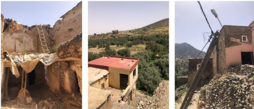
Figure 1.1. Ait Bourde partial destruction and severe damage
